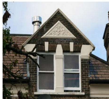
Visible flue from the streetscape
