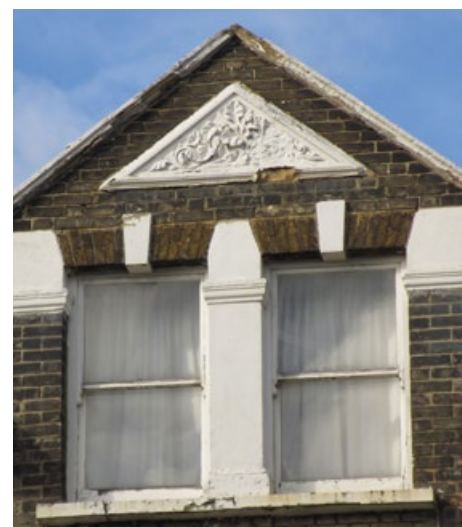
Historic plasterwork in need of repair
