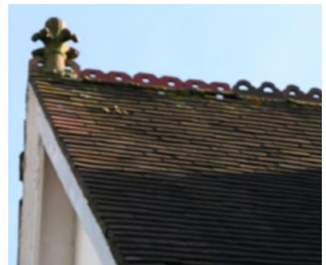
Poor repair of decorative roof tile
