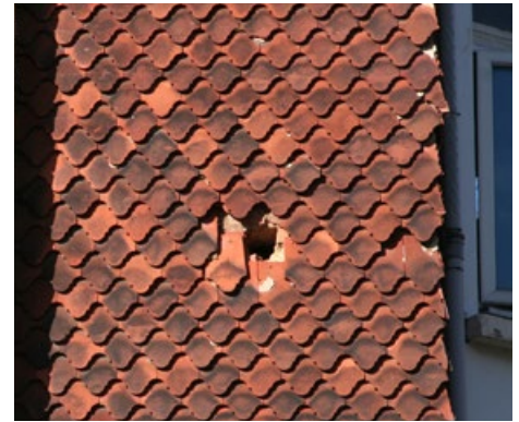
Hanging tiles in need of repair
