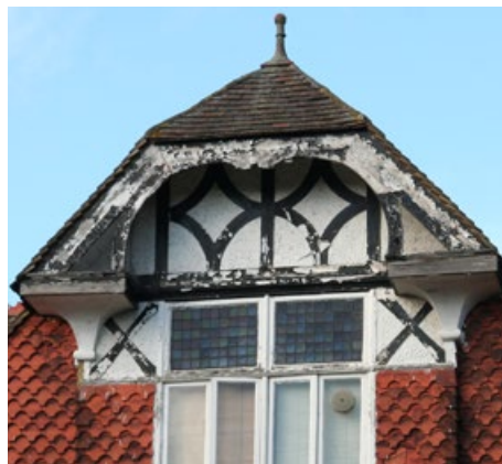
Poorly maintained timber bargeboard
